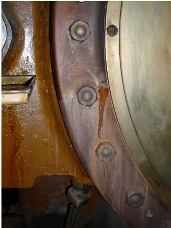
Figure 11. Cracked LP cylinder cover
