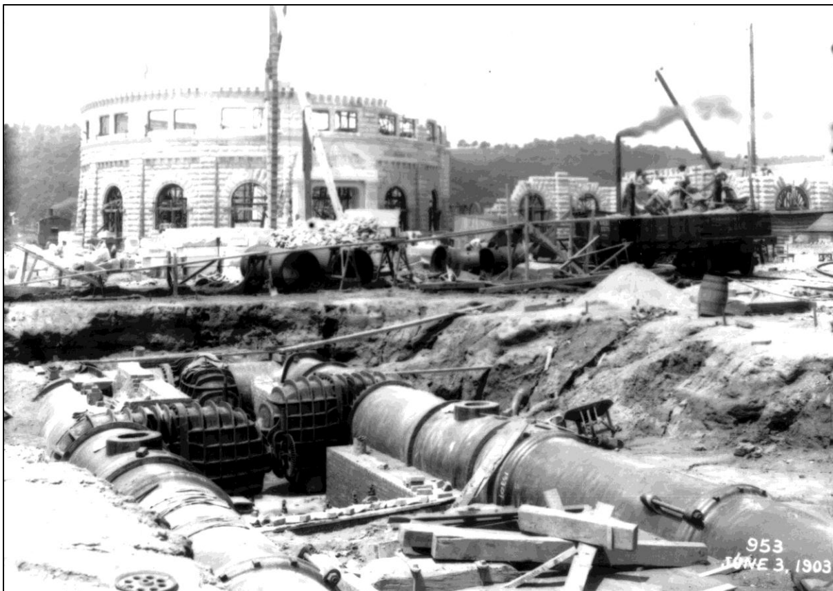
"New Works" pumping station for the Cincinnati Water Works under construction in California.
